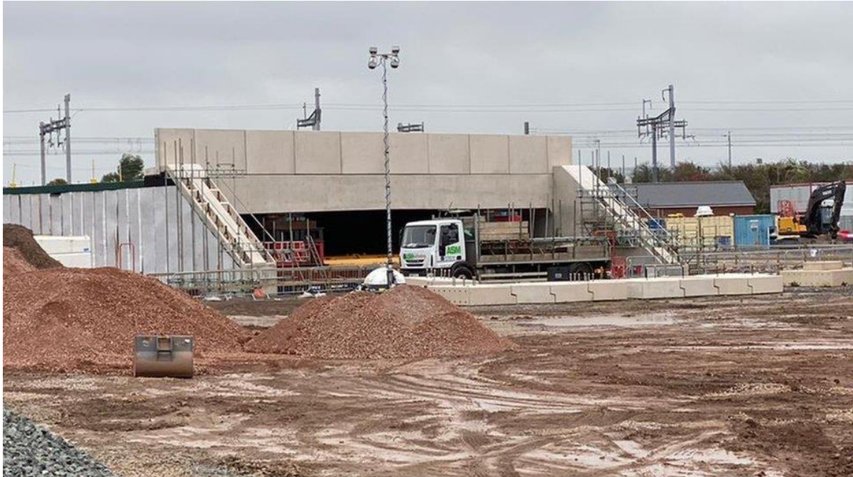
The new rail bridge will allow Gipsy Patch Lane to be widened
