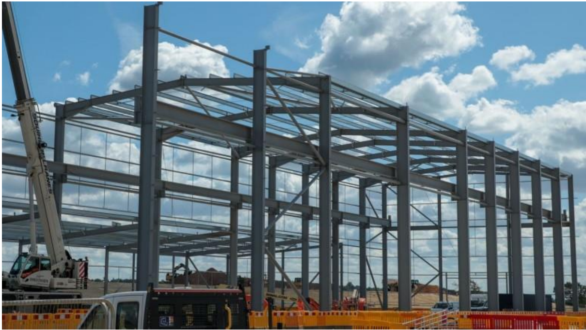
HS2's concrete plant at the Chiltern tunnel south portal site at Chalfont Lane takes shape.
