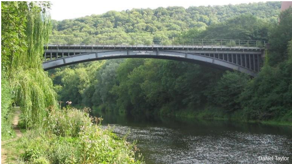
The Albert Edward bridge, which carries the railway over the River Severn, was designed by Sir John Fowler. (Shropshire Star)
