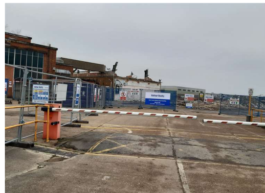
The view from the entrance, with just the boiler room still standing
