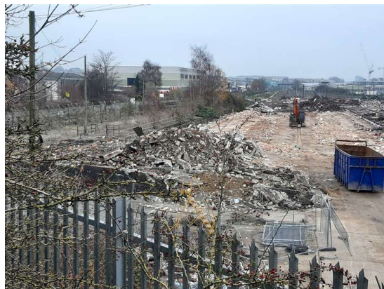
Piles of rubble close to the railway line
